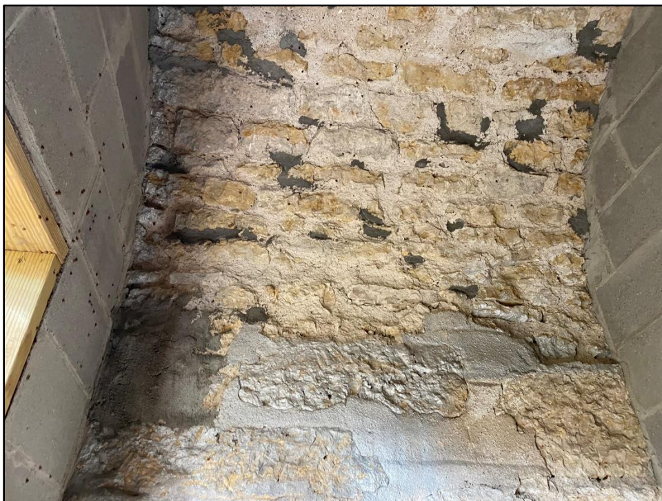
Photo 25: Different mortar at entry arch
