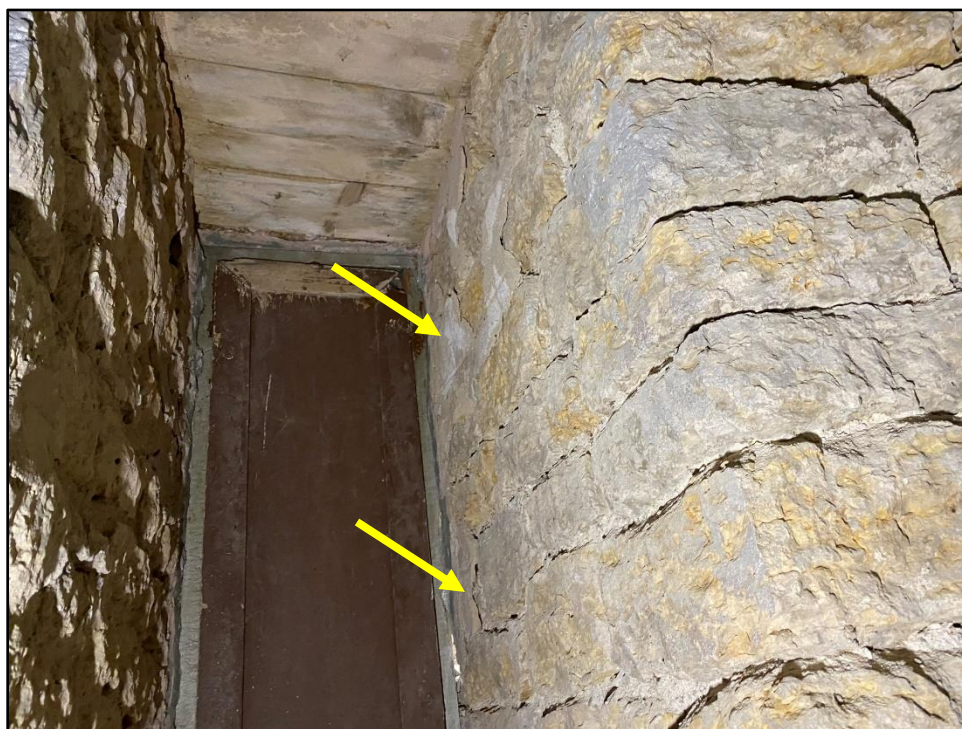
Photo 19: Spalled stone on “door” walls
