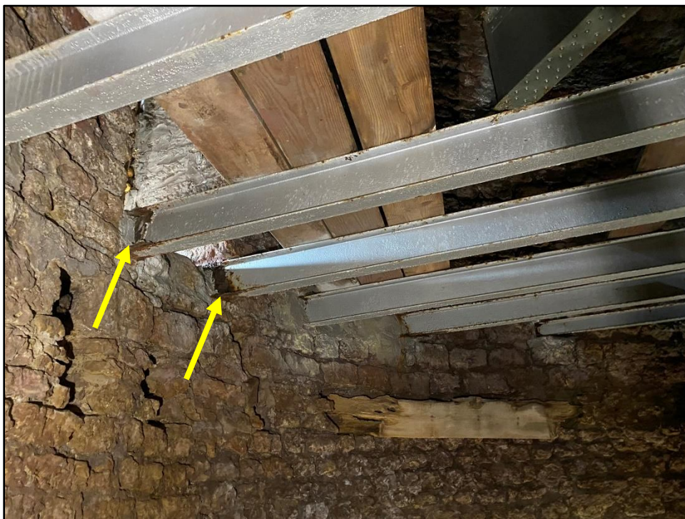
Photo 34: Signs of floor beam corrosion at walls
