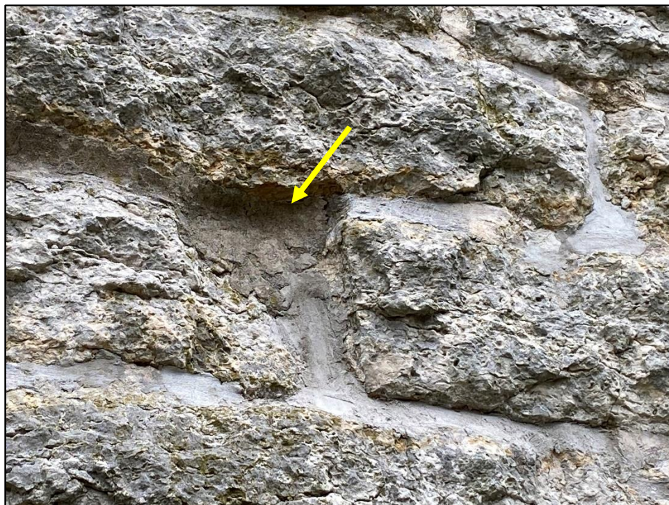
Photo 18: Isolated locations of stone spalls
