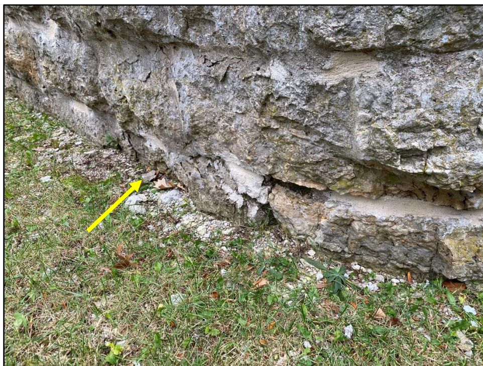
Photo 21: Stone deterioration at base of wall
