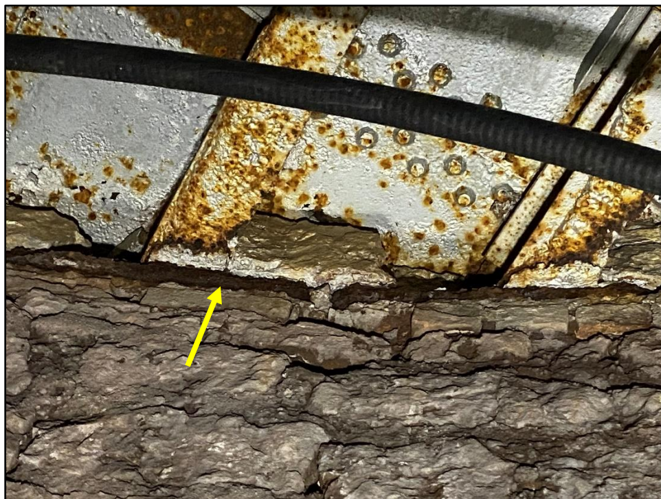
Photo 32: Close up of tank supports at wall
