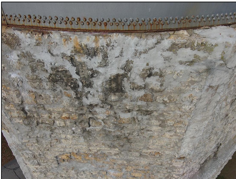
Photo 27: Repointing mortar at top of tower
