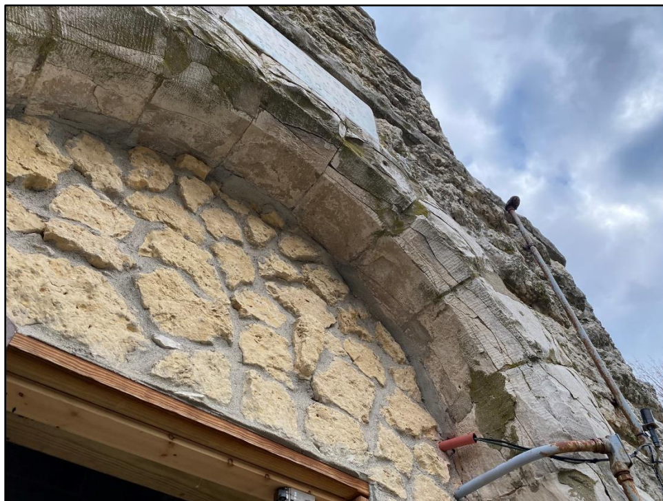
Photo 23: Cracked stone in entryway arch
